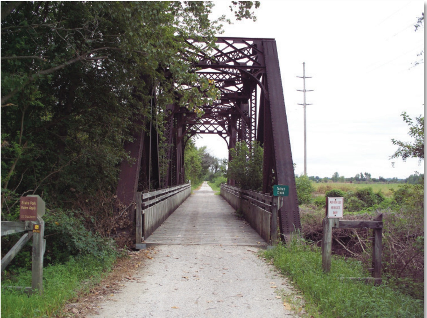
The Katy Trail Turkey Creek Bridge in Callaway County, across the Missouri River from Jefferson City.
